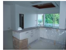
A5-3 Kitchen with recessed ceiling and air-conditioner ducting
