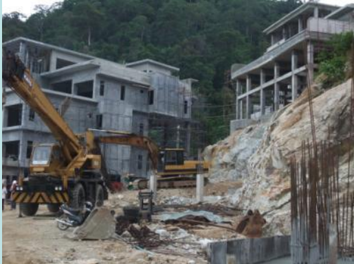
A3 at the back with building A2 building on top and phase C ground works in foreground
